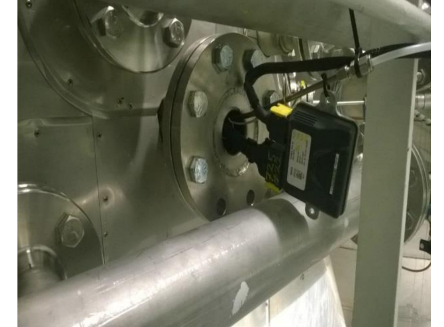
NH 3 sensor installed in stack
