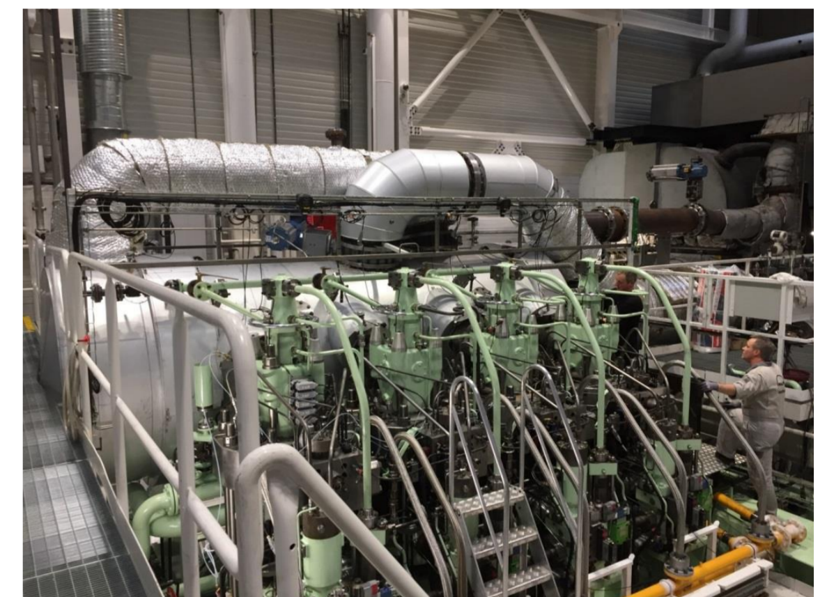
Integrated SCR receiver installed on a 4-cylinder two-stroke R&D test engine in Copenhagen
